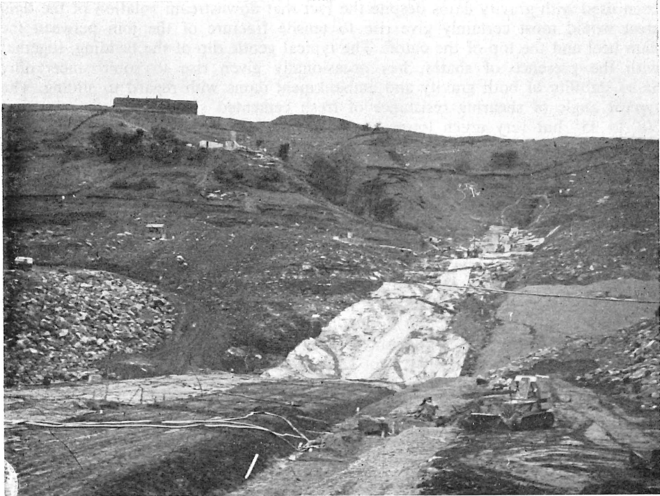
PLATE 5. — Left bank of Scammonden dam during construction illustrating core, filters and rockfill in foreground and cutoff zone in middle distance.
