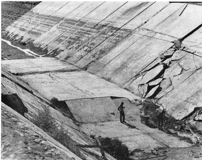
FIG. 11. — Prototype canal section several weeks after filling. The damaged canal lining had been placed on virgin soil, whereas the unbroken lining had been placed on soil which had been presubsided prior to excavating the canal prism.
