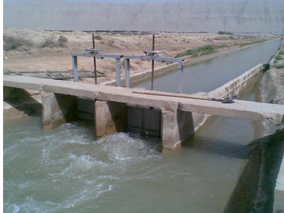
Figure 1. Two parallel sluice gates (Omidieh irrigation network located at south of Iran)
